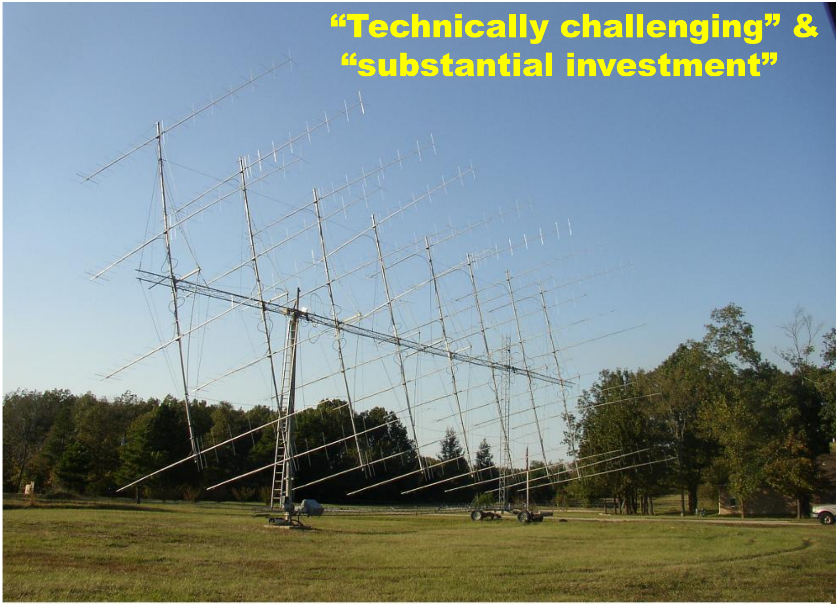
W5UN EME Array with 32 2M5WL horizontal antennas, and 32 front mounted ten element vertical antennas
